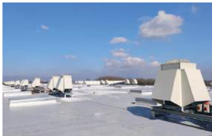
Halms csarnok, Debrecen - 22 pcs Hoval TopVent® TP recirculation units with heat pumps
