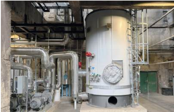
Power Plant, Tatabánya - 1 pcs 20 MW Parat electrode boiler
