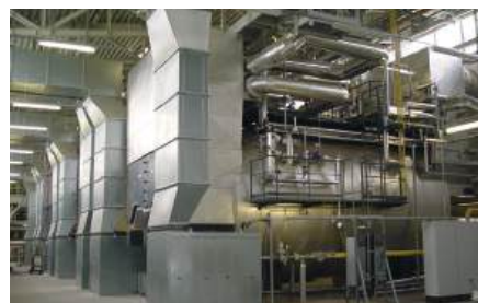
Dunapack Zrt., Dunaújváros - 4 pcs astebo THD-IZ steam generators (55 t/h)
