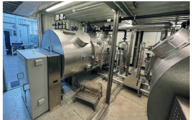
Aluminum extrusion plant - 2 pcs Ecotherm elektromos steam boilers (1500 kg/h) in container design
