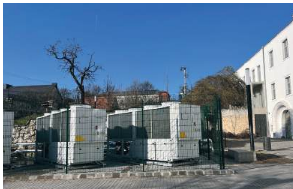
Premontrei Order, Gödöllő and Zsámbék - 6 pcs Enerblue heat pumps, 3 pcs Hoval buffer storages and 3 pcs hot water tanks
