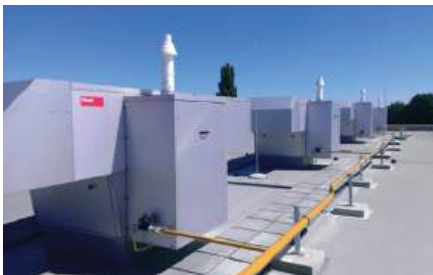
Schott Hungary Kft., Lukácsháza - 10 pcs Hoval TopVent®, 4 pcs Hoval RoofVent® condens
