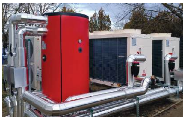
Primavet Produkt Kft., Budapest - 3 pcs Hoval Belaria® fit heat pumps, 2 pcs Hoval TopGas® gas boilers, Hoval CombiVal E buffer storage
