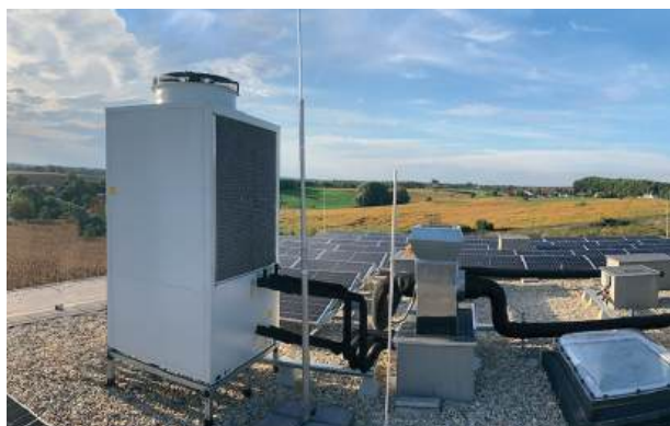
Gébárti Lakópark, Zalaegerszeg - 3 pcs Enerblue Orange HT eat pumps, 3 pcs Hoval buffer storages, 3 pcs Hoval hot water tanks
