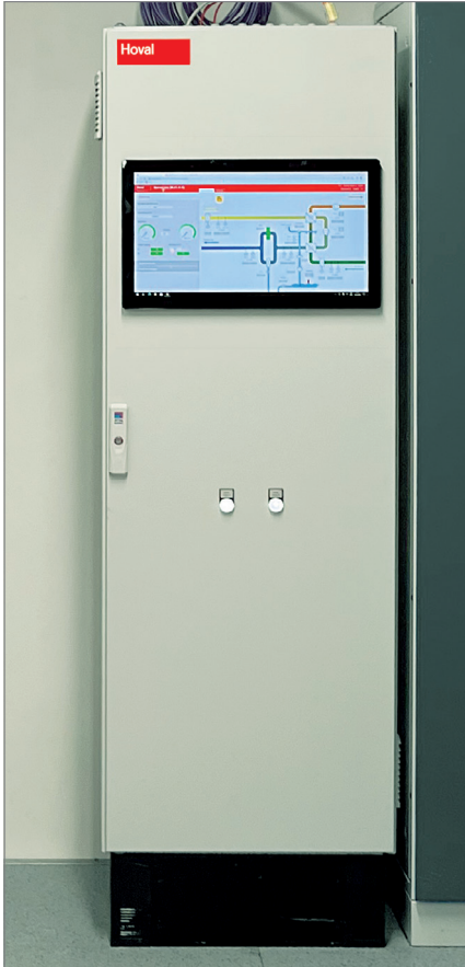
Fig. D3: Zone control panel
